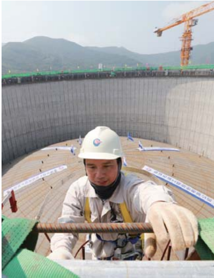
▲ During the pneumatic jacking process of the storage tank, the construction workers went to monitor
